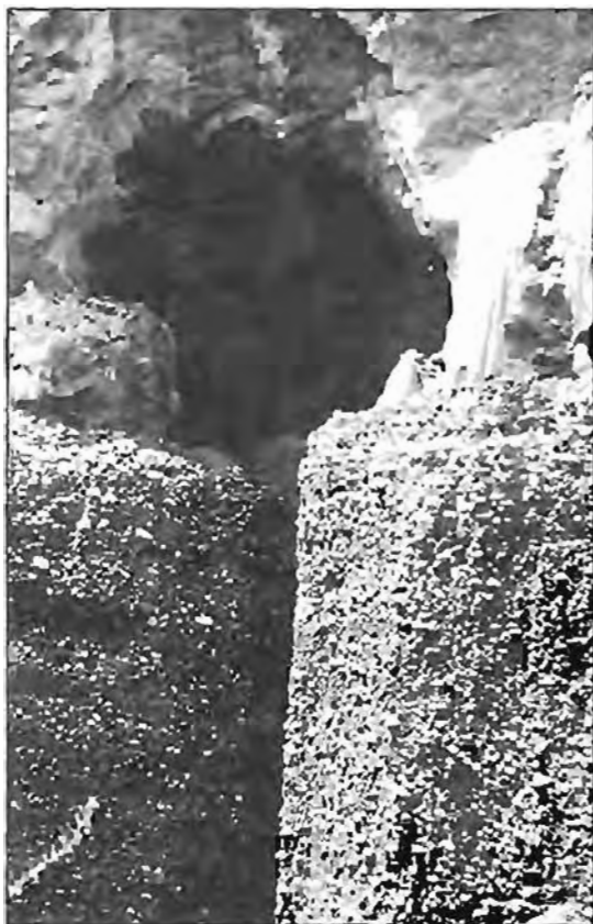
FIGURE 5. Erosion tunnel at the contact of two layers of Cretaceous soils in excavation at the Bouldin damsite. Note the vertical joint in the cohesive gravelly material.
